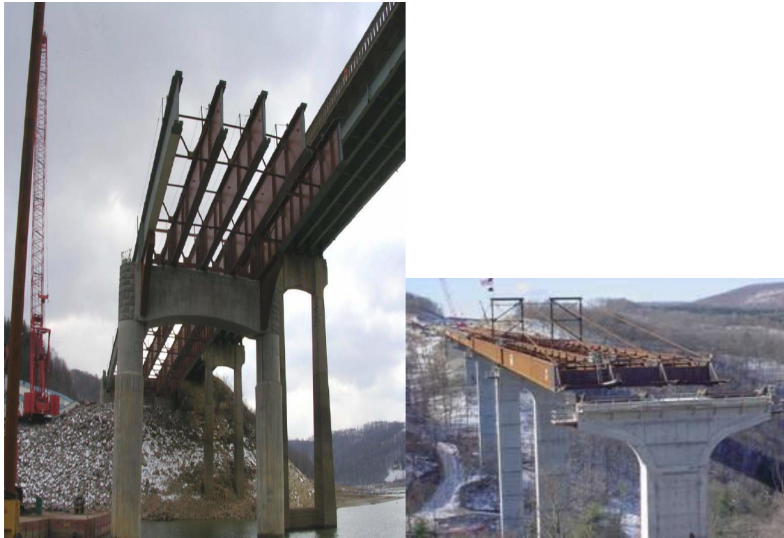
Figure 8 Girder Erection by a Crawler Crane and Also by Incremental Launching with Cable Tie-Backs.
