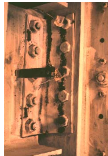
Figure 2.5. Failure of Angle
