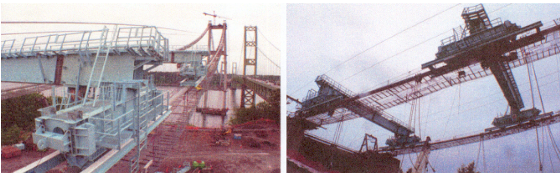
Figure 4.5.1: Two photos of the Tacoma Narrows Three Bridge lifting device built by a Korean firm
